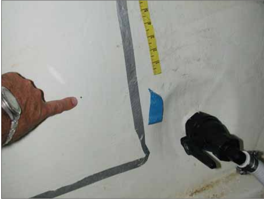
A core closeout for a lightweight Marelon composite fitting and valve, built into a vacuum-bagged, wet-preg, cored hull. Note the concentric laminate patches and their offset darts.
