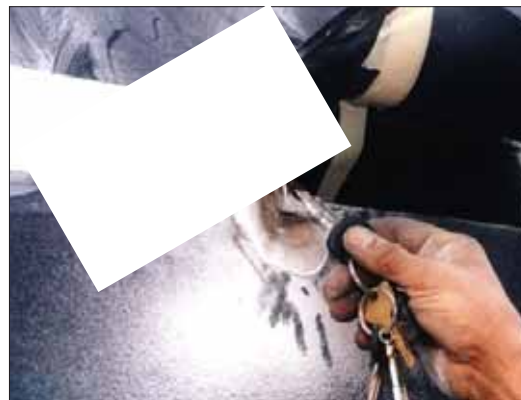
Scuppers and drains should be treated the same way as cored-panel penetrations below the waterline. This scupper tube was laminate-taped on the inside, but only puttied and painted on the outside. After five years in service, it was surrounded by a wide margin of wet and rotted core.
