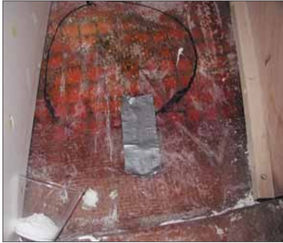
The water in the core kerfs of this large motoryacht developed an unpleasant smell and blackened the PVC foam core in less than 18 months. Shown here is a leak into the master head's vanity at a self-tapping screw location.
